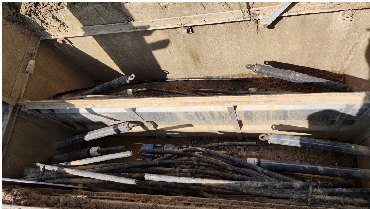
Exhibit 12: Fiber optic cables cut in several locations in France prompting an criminal investigation (Source: CYBERSCOOP)
